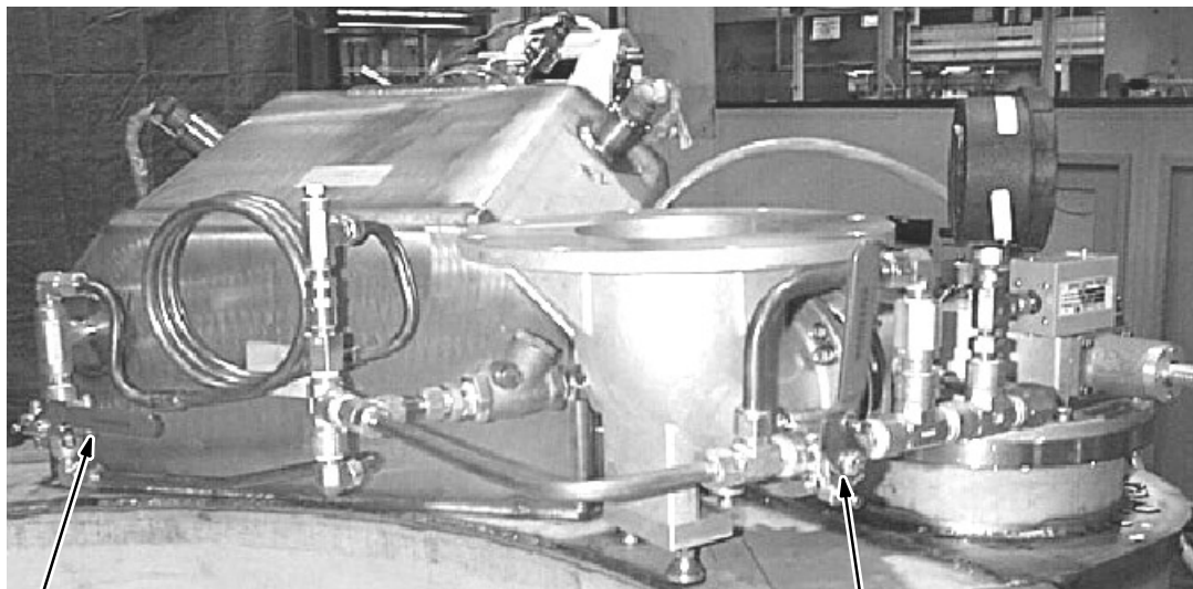
SHIELD COIL EXHAUST VALVE ( V3 )
