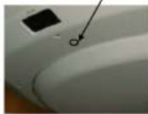
Old Ceiling Cover
