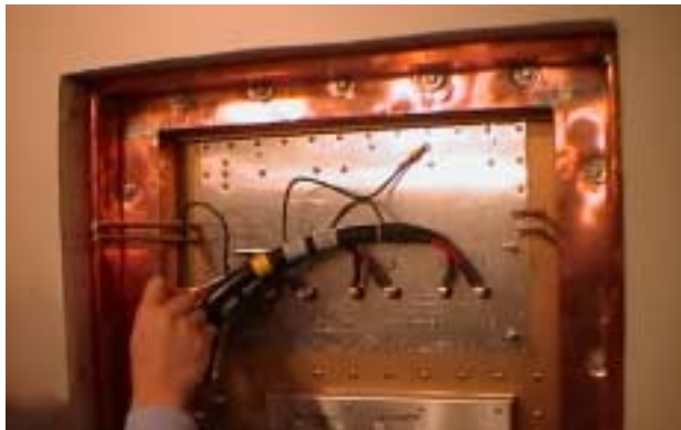
GRADIENT CABLE CONNECTION (SCAN ROOM SIDE) ILLUSTRATION 2
