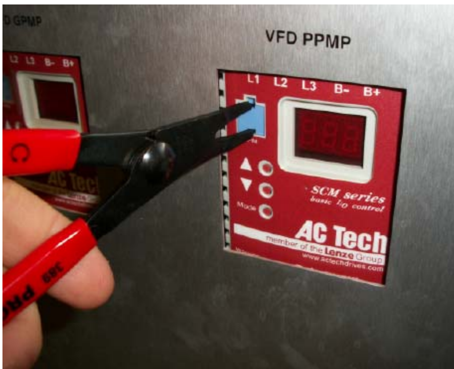
Figure 6 Remove the existing VFD chip with replacing the Ebara pump with a Price Pump.
