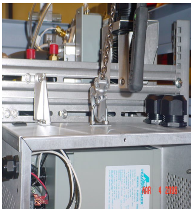
Picture 3 Hoist attachment to Power Box
