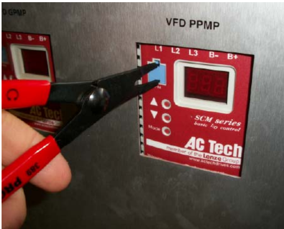
Figure 6 Remove the existing VFD chip with replacing the Ebara pump with a Price Pump.
