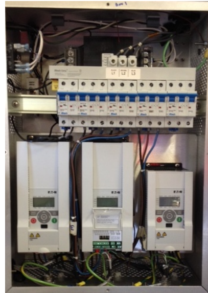
New Eaton Box Uncovered
