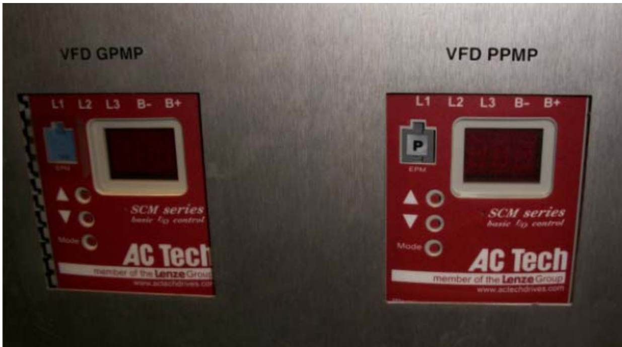
Figure 7 Complete installation. (This HEC has an Ebara gradient coil pump and a Price power electronics pump, as noted by the 'P' on the VFD chip in the power electronics VFD)
