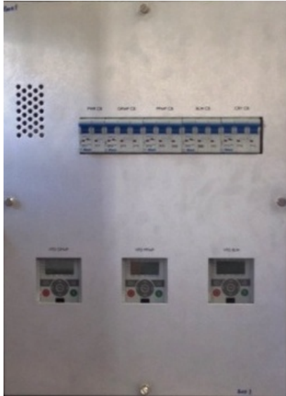
New Eaton Box Covered
