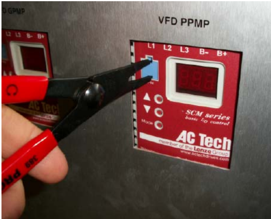
Photo 7 Remove the existing VFD chip with replacing the Ebara pump with a Price Pump.
