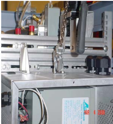
Figure 3 Hoist attachment to Electrical Box
