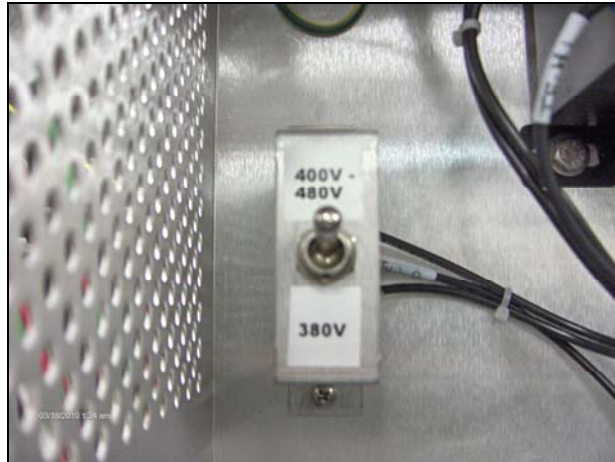
Figure 7: System 380/400-480V Switch
