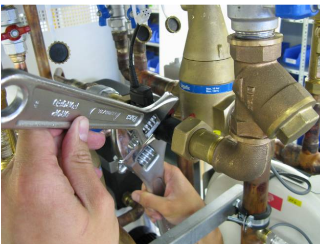
Figure 77 – Primary flow and temp sensor
