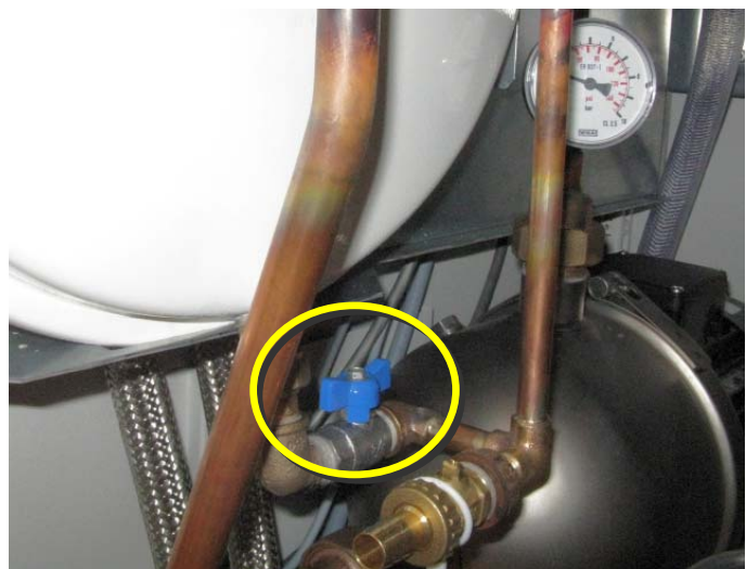
Figure 16 – Valve of expansion vessel
