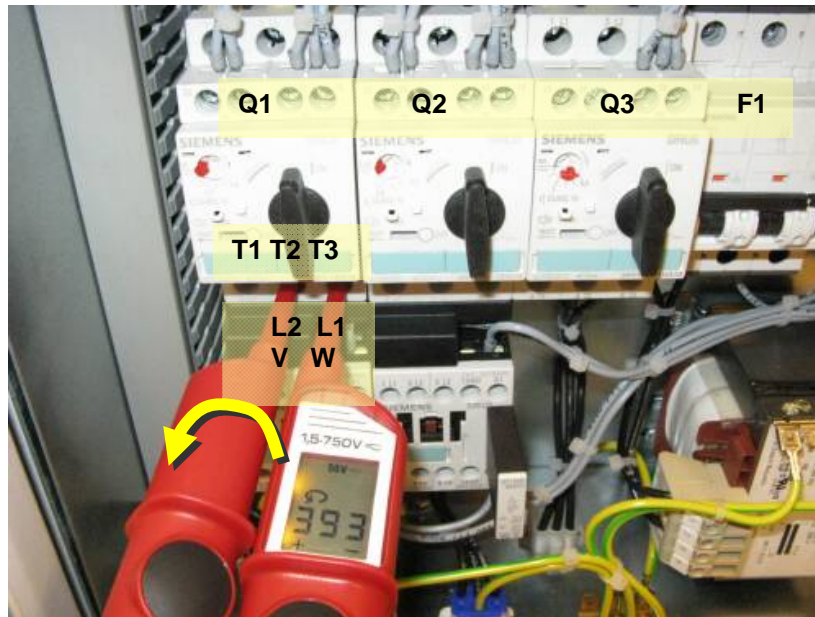
Figure 8 – Measure in the electronic box
