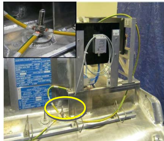
Figure 4 - Central PE of the Magnet
