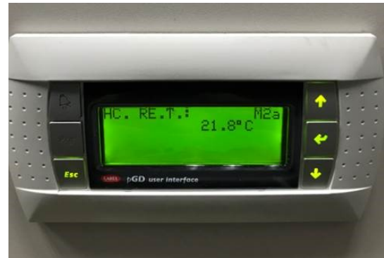
The HC return temperature shows in °C.
