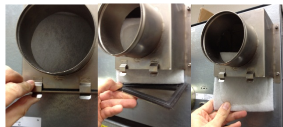
Figure 7 – PVU filter replacement
