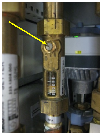
Figure 13 - Locate the RF amplifier flow setter
