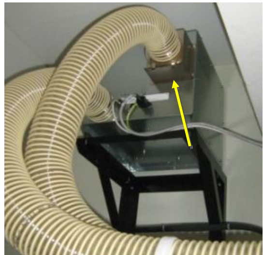
Figure 6 - Patient ventilation unit-air-inlet
