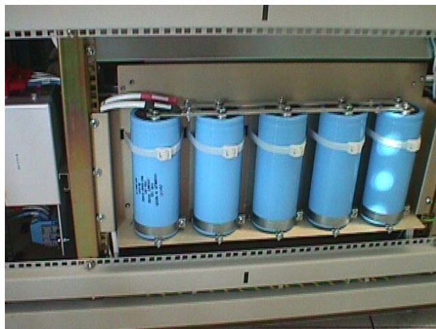
Figure 12 - buffer capacitors in the cabinet
