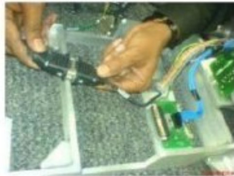
Connection Table control Board Cable
