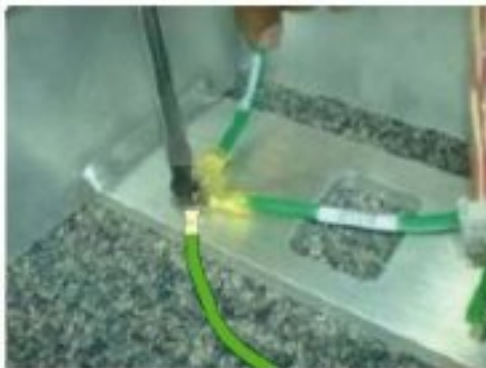
RUN#M4503 Connection Earthing Cables.
