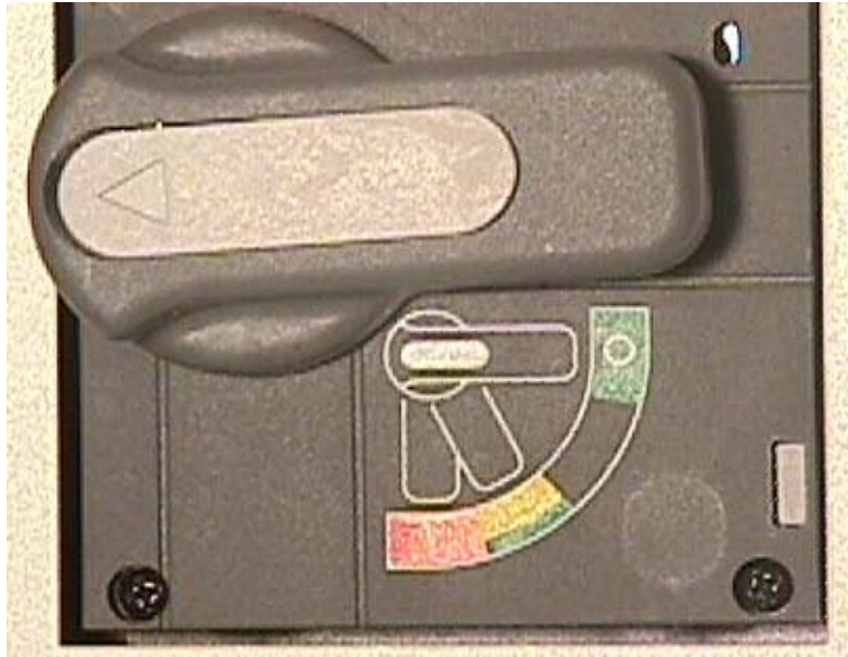
MAIN INPUT BREAKER IN THE OFF POSITION ILLUSTRATION 2-2
