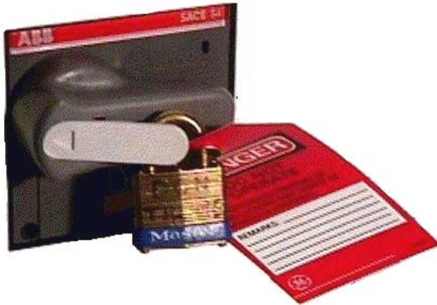
PDU MAIN INPUT CIRCUIT BREAKER LOCKED AND TAGGED OUT ILLUSTRATION 2-3
